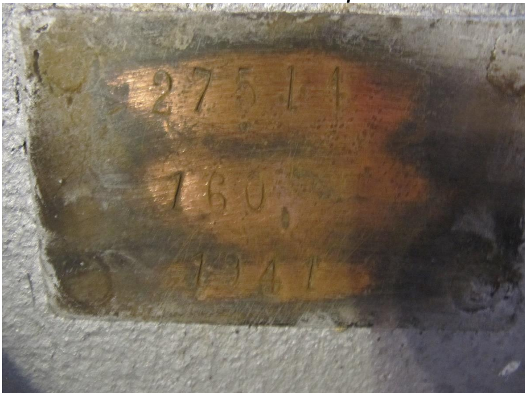
Boiler plate of 'SINEMBE'. Riverside September 2010
