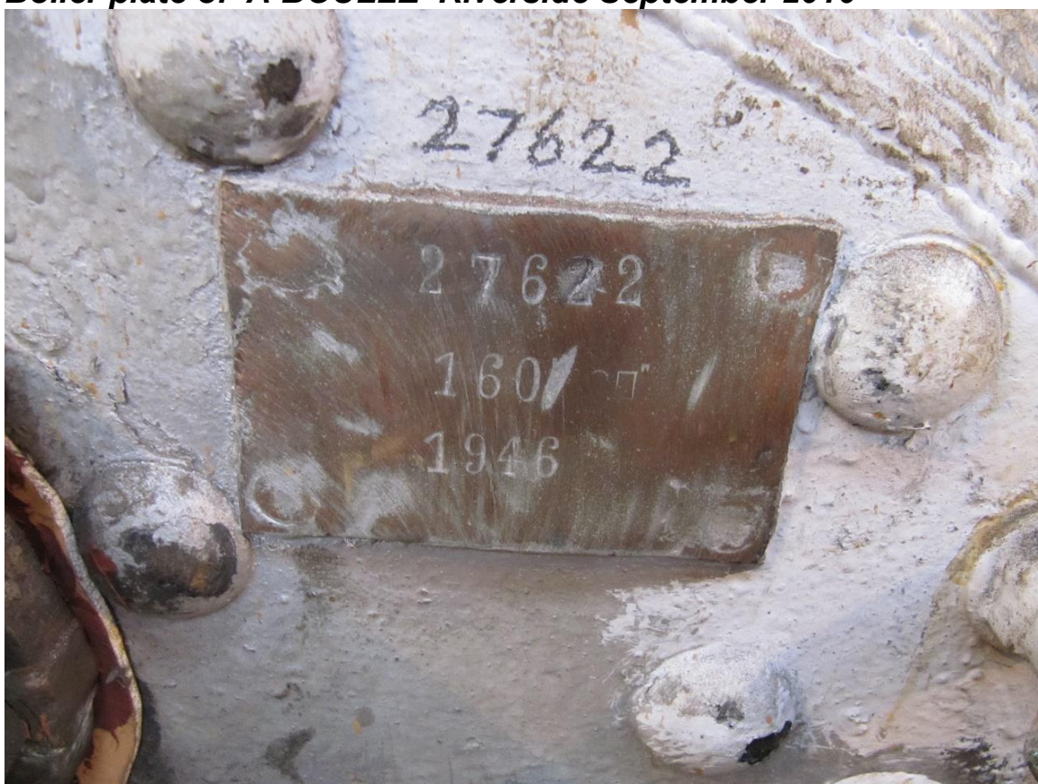
Boiler plate of 'CHARLES WHYTOCK' Riverside September 2010 This was the original boiler which it seems to have kept its entire life.
